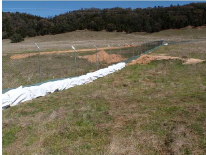
Photograph 3. Silt trap at the southern boundary
