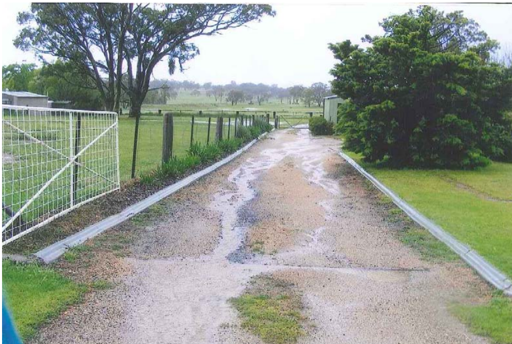
■ Figure 2-4 Stormwater running along the Driveway of 15 George Street
