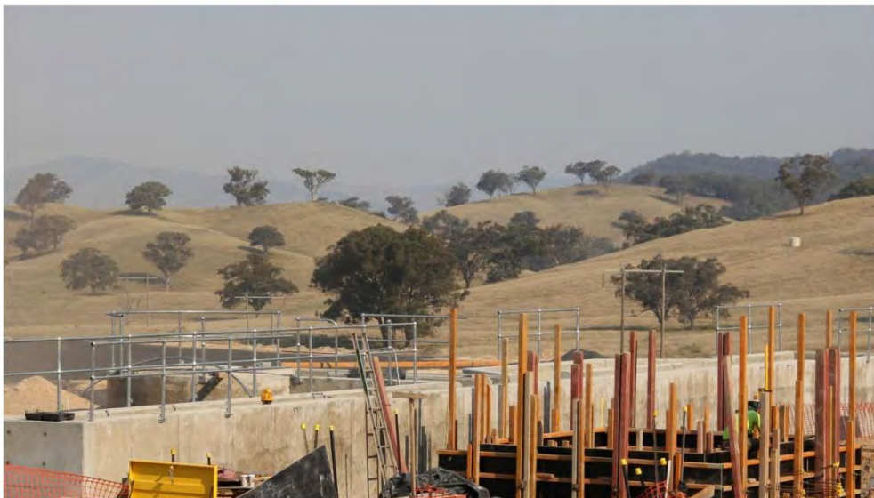
Photograph 2. Concrete works complete and handrail installed at inlet works. Construction of formwork for septage receiving facility.
