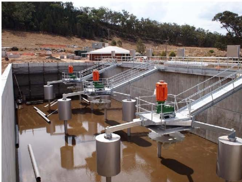
Photograph 2. Aeration equipment installed in aeration tanks
