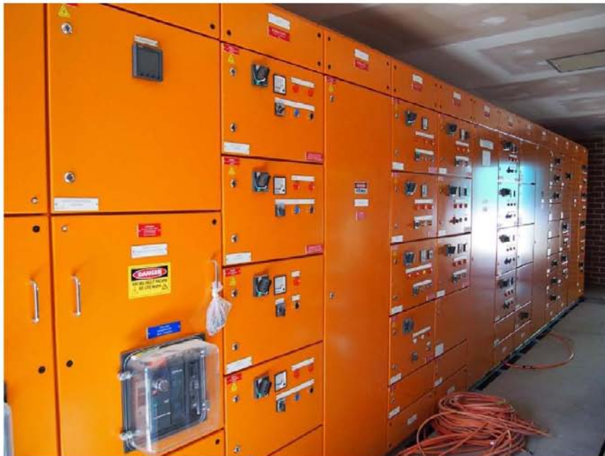
Photograph 1. Main switchboard installed in switchroom.
