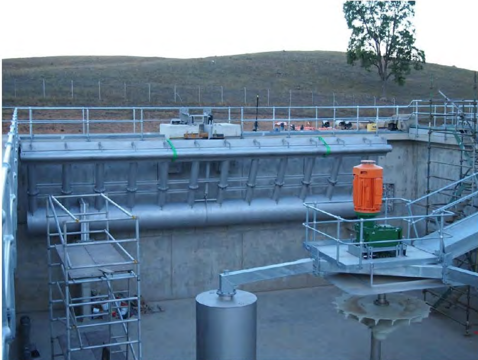
Photograph 1. Mechanical decanter installation.
