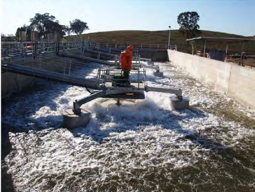
Photograph 1. Aerators operating during testing.
