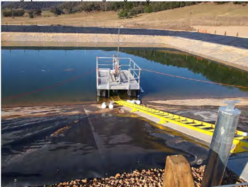
Photograph 2. Mixer installed in sludge lagoon.
