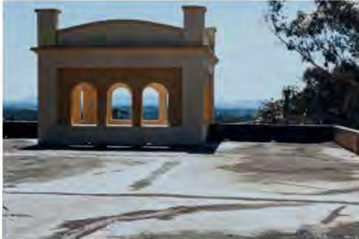
Figure 7: The original flat roof of the museum, now covered over with a pitched metal lined roof. (Dept of Environment image- copyright)
