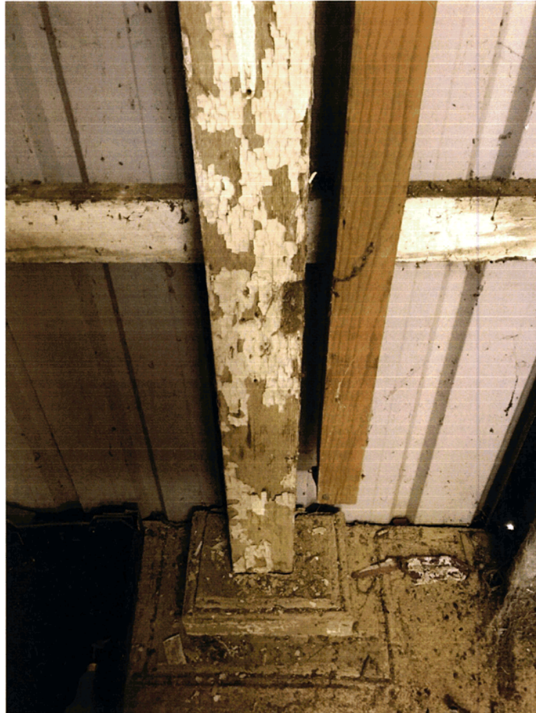
Photo No.4 – Termite damage to C1 and C2
