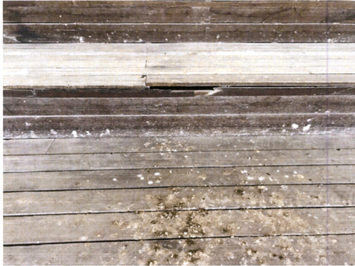
Photo No.6 – Weathering/splitting of seat boards B7
