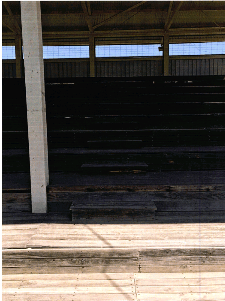
Photo No.7 – Non-compliant stairs
