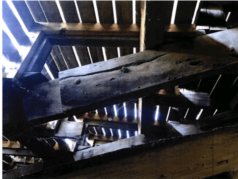
Photo No. 3 – Failed splice joint of B1
