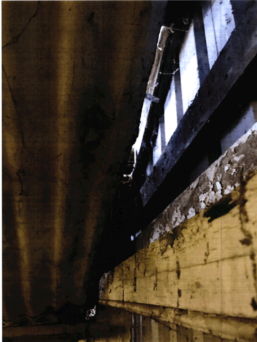
Photo No.5 – Termite damage to end wall girts
