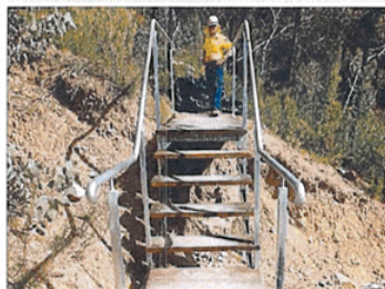
The Fan's Horizon track reopened this week following the replacement of around 1,000 timber steps, marking the full recovery of the Warrumbungle National Park.
