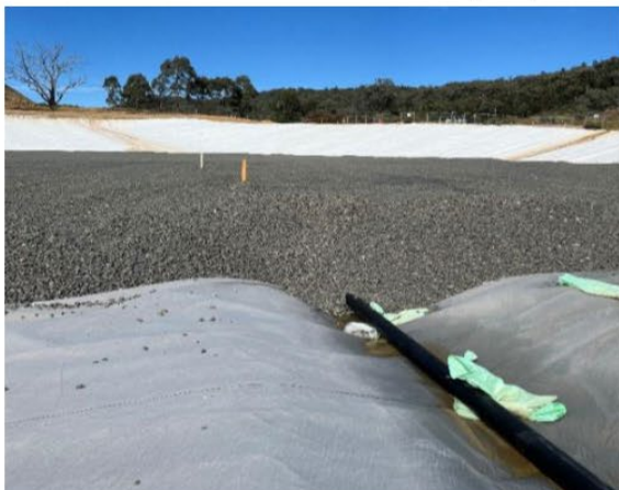
Aggregate drainage layer leachate drainage system
