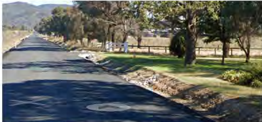
Above: Swale drainage at the front of 34 Bruce Road which runs along the length of both sides of Bruce Road and onto Springs Flat Road.
