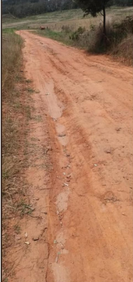
Figure 13 Poor Road condition approx. halfway along the proposed 125m
