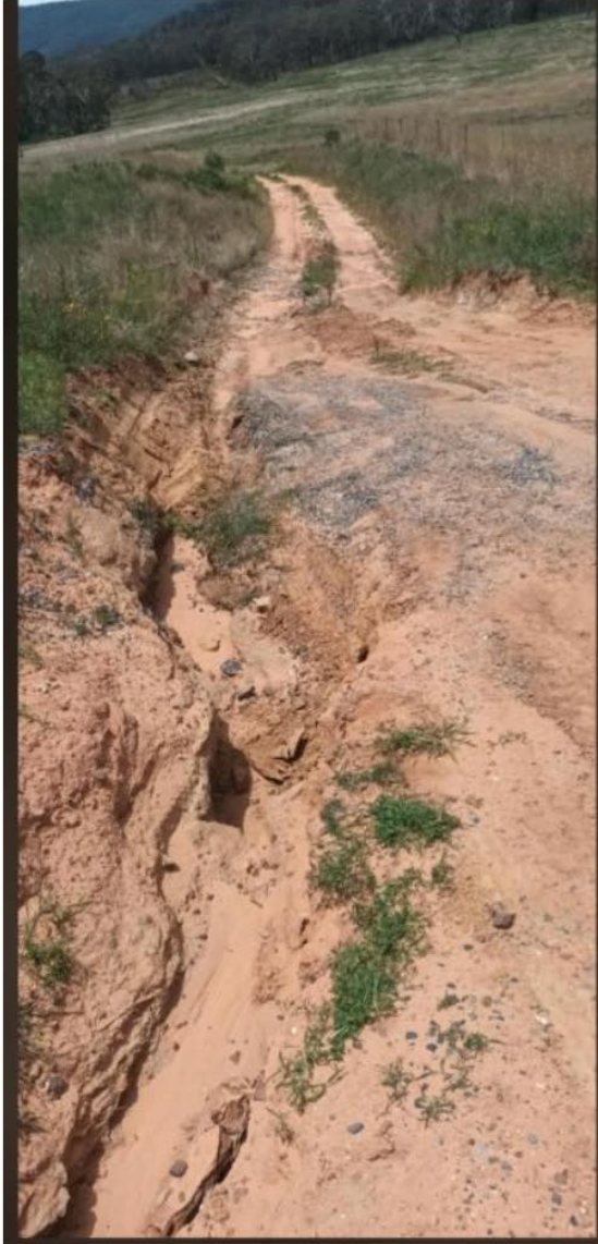
Figure 14 Significant damage to road in front of new access way for residence and carriage way. This is unpassable at times preventing the lots further on access and preventing access to State Forest
