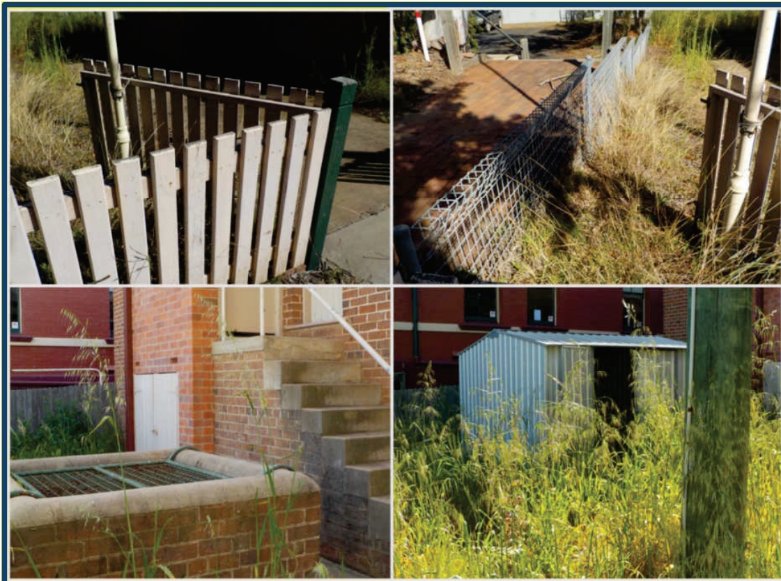
Figure 17 - Fire Station External Assets (Clockwise top LHS) boundary picket fencing and gate, fencing and path, garden shed and rear of Fire Station.
