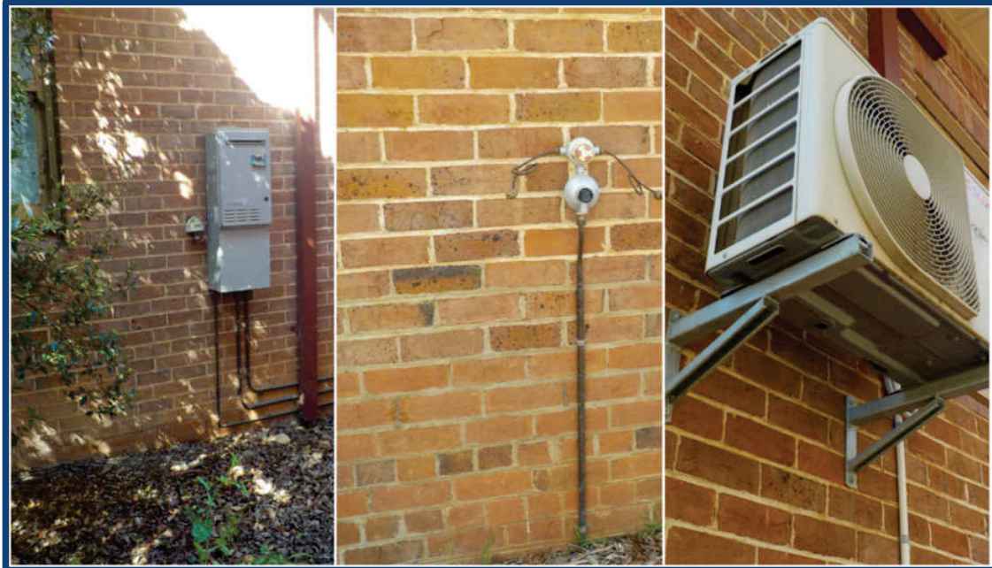
Figure 16 - Fire Station Installations
