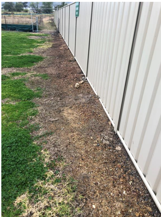
Figure 5.6: Bare soil next to existing facility fence.
